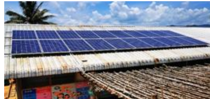
Solar Cell System 5.3kWp
