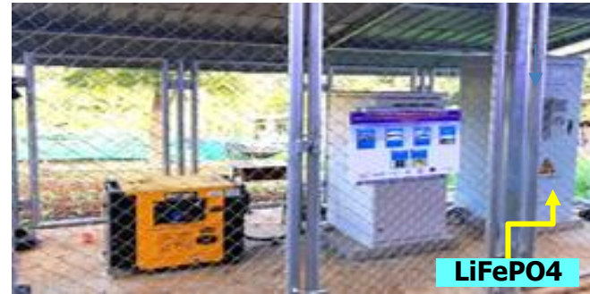
Solar Power & Battery Cabinets
